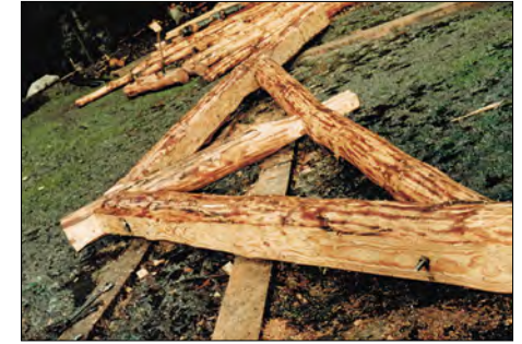
One of the big log trusses that we used in the café. They were bolted together in the carpark and then carefully manoeuvred into place using a lever and the front end loader of an old David Brown tractor
